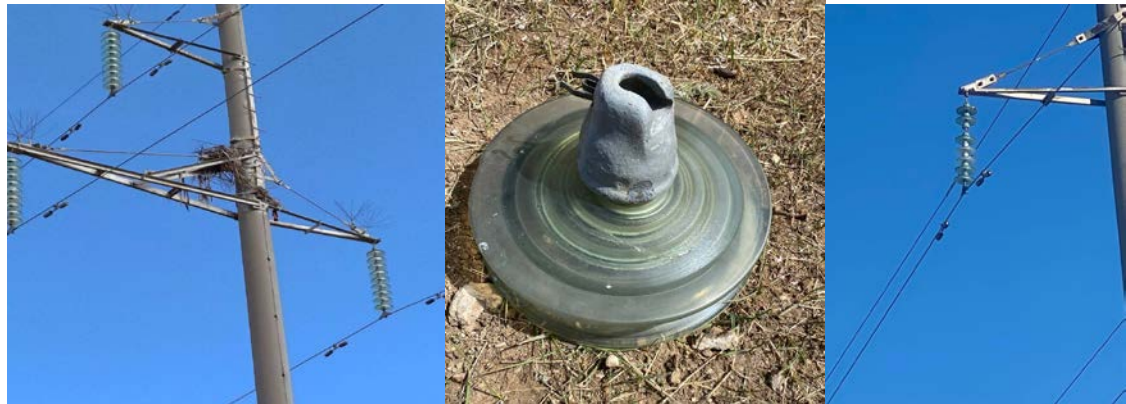
Fig. 4 Pole power line with concrete support is broken due to external factors
